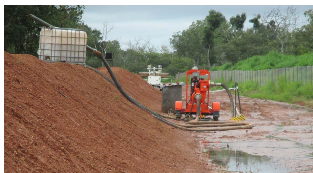
Basin overflow and pumping attempt, August 2018
