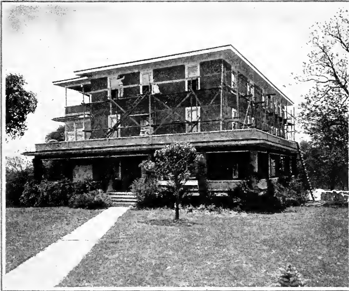
Hospital Buildings No. 1 and No. 3 The Nurses' Home. Additional Story under Construction
