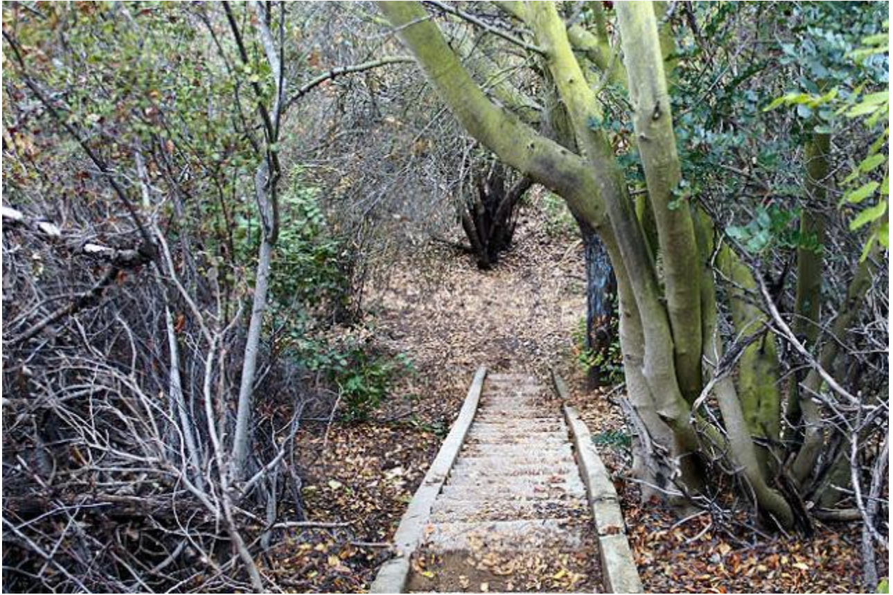
The end of the line for the stairway leading to the floor of Rustic Canyon.
